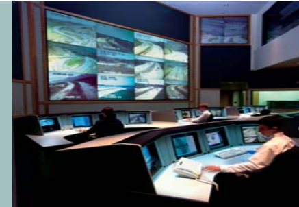
The CommuterLink Control Center
