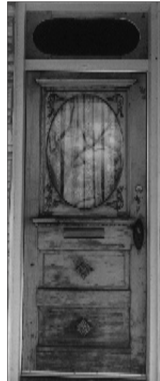
When a historic door or its components are damaged, repair them and maintain their general historic appearance.
