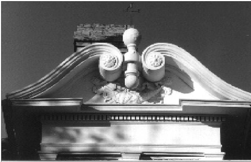
Features such as window hoods, brackets and columns are often associated with particular styles and therefore their preservation is important.
