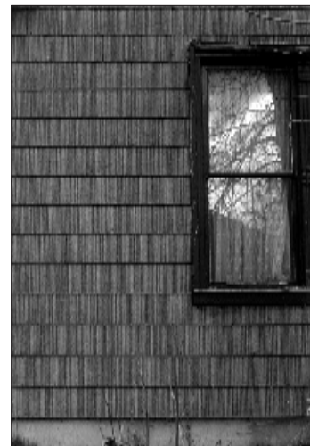
Inappropriate: These shingles cover original wood siding. Using any material, either synthetic or conventional to cover historic materials, is not allowed. Doing so would obscure the original character and change the dimensions of walls, which is particularly noticeable around door and wood openings.
