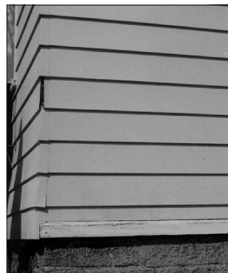
This metal siding covers original wood clapboards. Using synthetic material to cover historic materials is not allowed.
