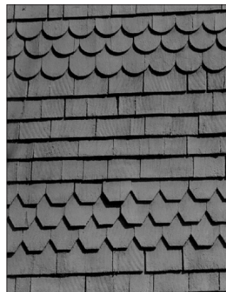
Decorative wood siding should be preserved.
